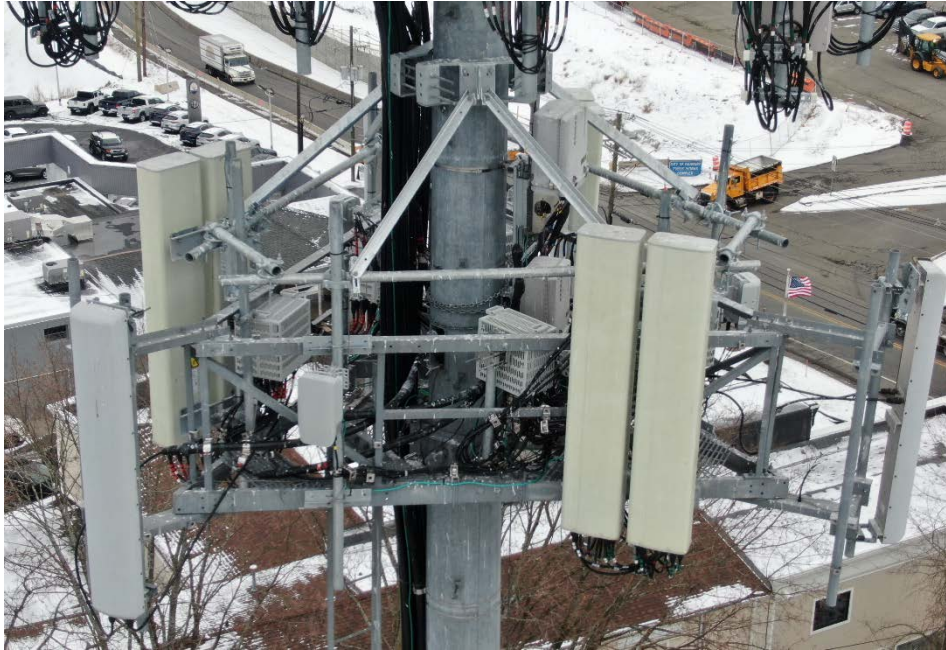
Photo 1: Photo illustrating the monopole with Appurtenances shown.
