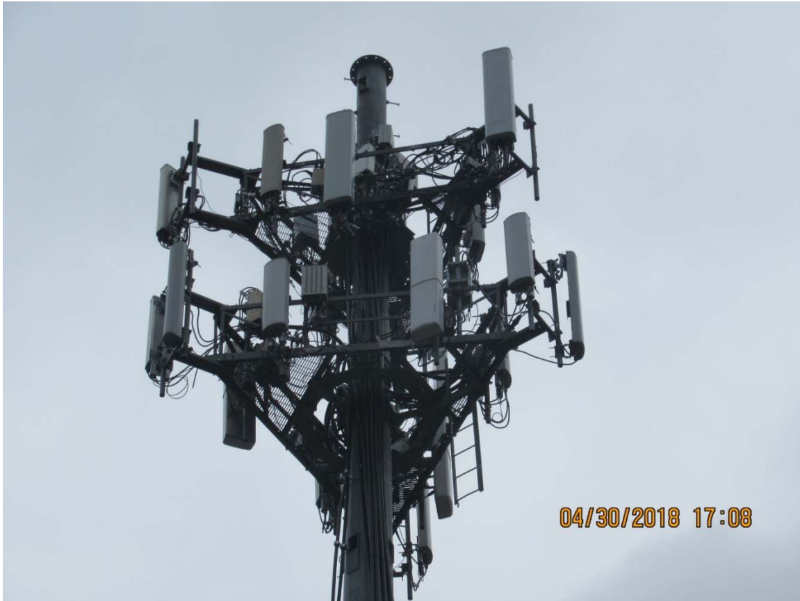
Photo 1: Photo illustrating the monopole with Appurtenances shown.
