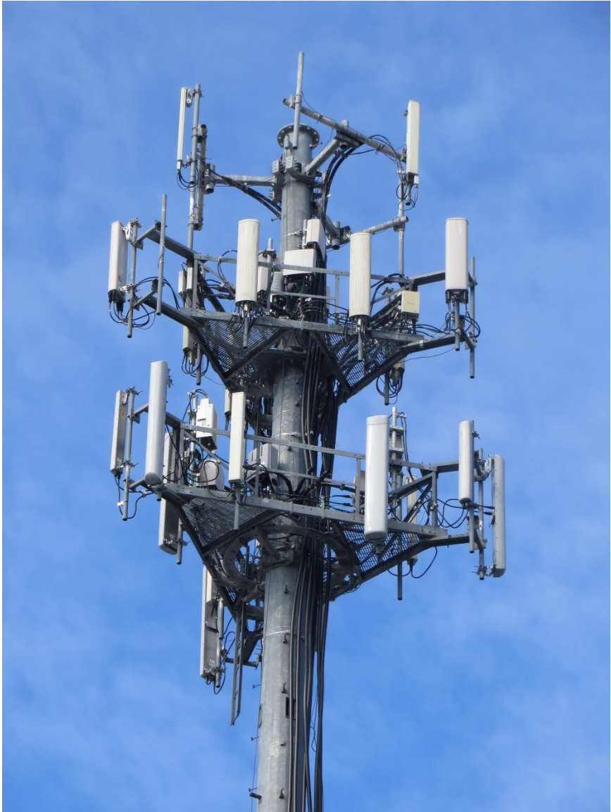
Photo 1: Photo illustrating the monopole with Appurtenances shown.
