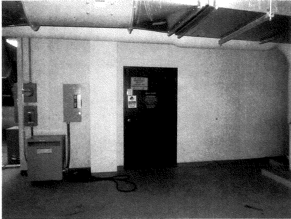
Figure 8: Verizon Equipment Shelter
