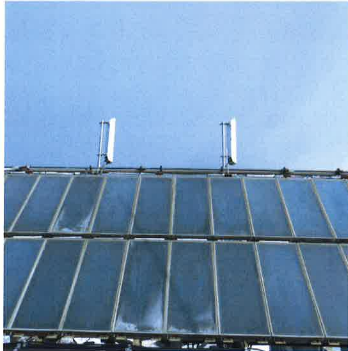
Photo 1: Sample photo illustrating the existing T-Mobile antennas.
