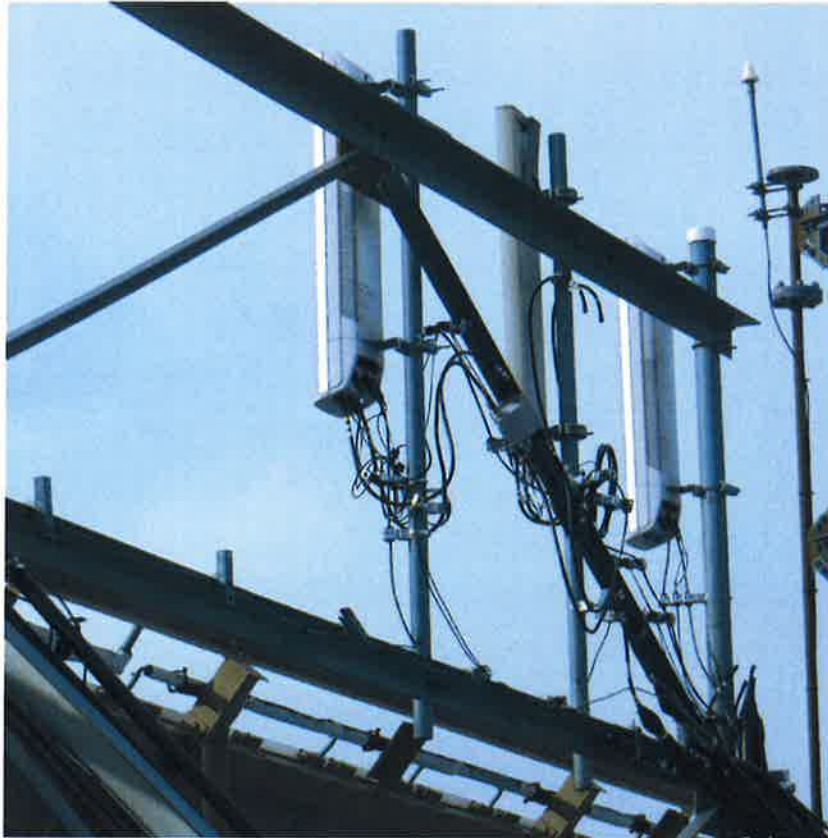
Photo 3: Sample photo illustrating the existing T-Mobile antennas.
