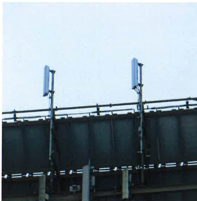
Photo 2: Sample photo illustrating the existing T-Mobile antennas.
