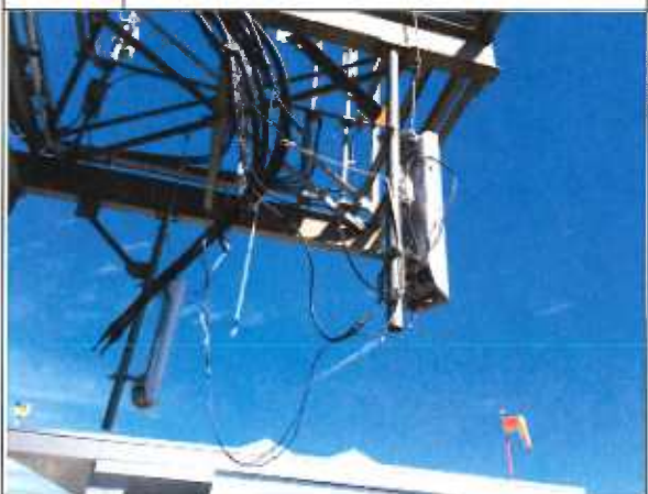
9. T-Mobile Sector A antennas
