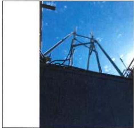
16. Verizon Sector B antennas, 1 of 2
