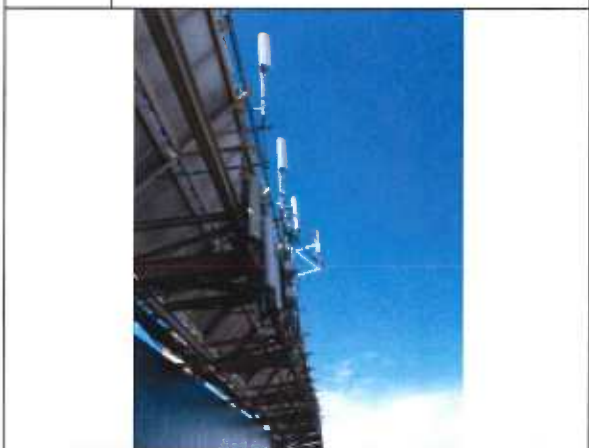
8. T-Mobile Sector B antennas and Sprint beyond
