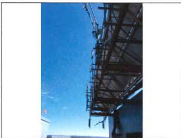
10. Sector A antennas
