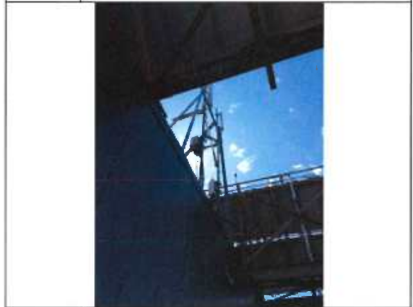
17. Verizon Sector B antennas, 2 of 2
