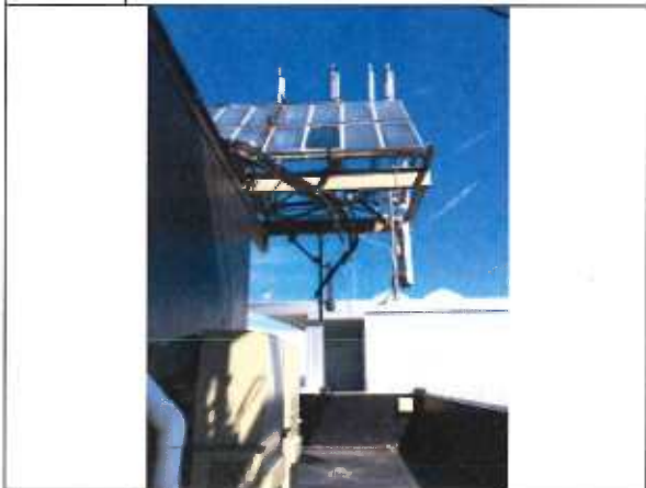
6. Verizon Sector A antennas above and T-Mobile Sector B antennas below
