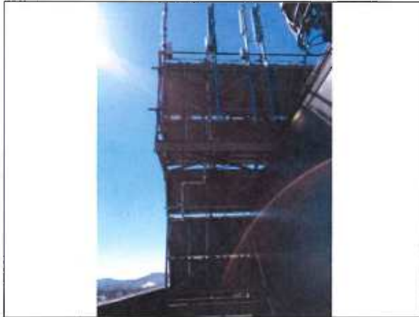
1. Verizon Sector B antennas
