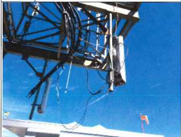
9. T-Mobile Sector A antennas
