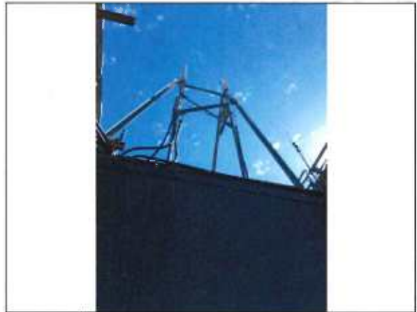
16. Verizon Sector B antennas, 1 of 2
