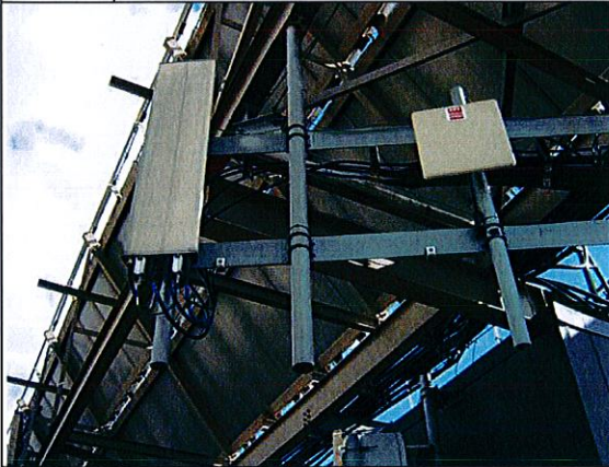
14. T-Mobile Sector A antennas (2 of 4)
