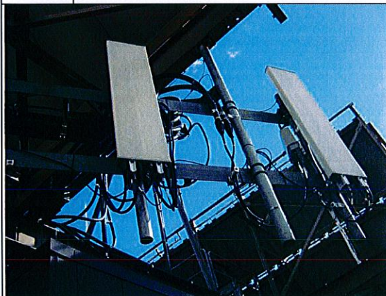
15. T-Mobile Sector A antennas (2 of 4)
