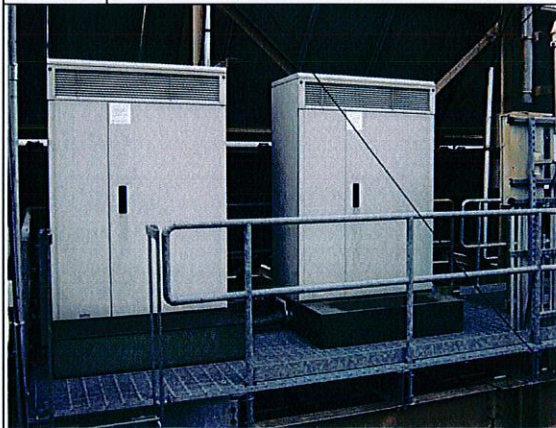
26. T-Mobile equipment on upper roof
