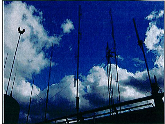
28. Antennas on upper roof
