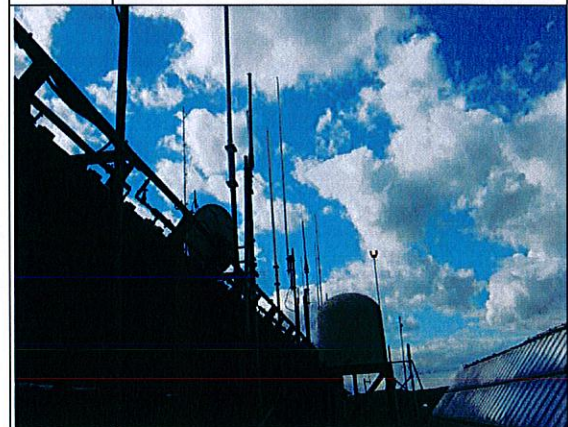
30. Omni and whip antennas on upper roof
