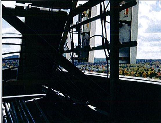
2. Nextel antennas (disconnected) on east wall
