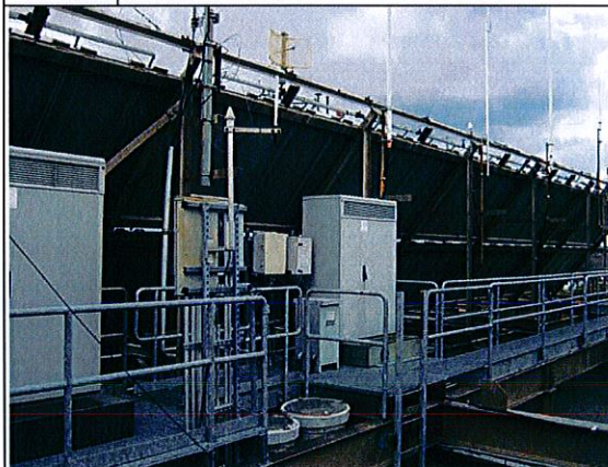
27. T-Mobile equipment on upper roof
