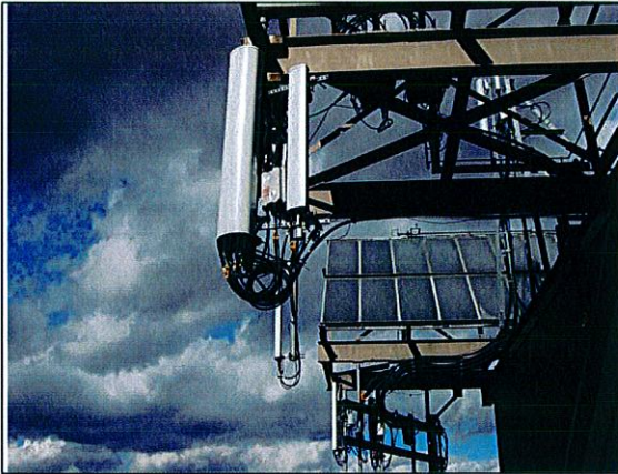
7. Sprint antennas on east side of building
