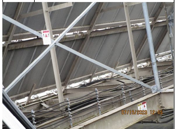
10. T-Mobile Sector B and D with Existing Signage
