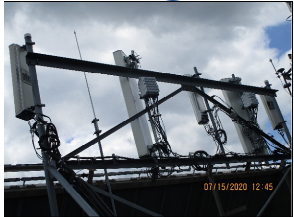
8. T-Mobile Sector B and D with Existing Signage
