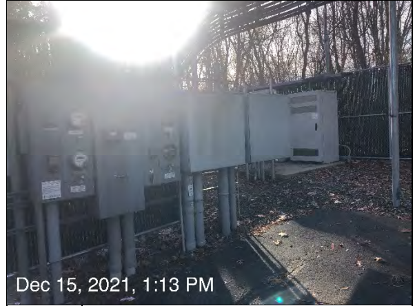
22. Equipment Inside Monotree Compound
