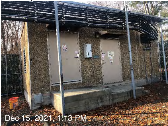
20. Other Carrier Equipment Shelter
