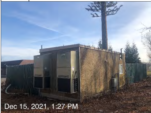
21. Other Carrier Equipment Shelter
