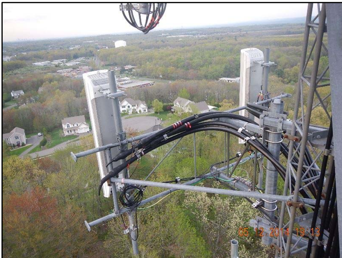
Existing T-Mobile Antenna Sector Mount on Tower
