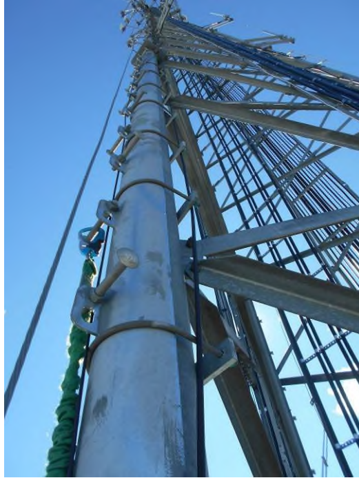
Photo of existing step bolts and safety climbing cable.
