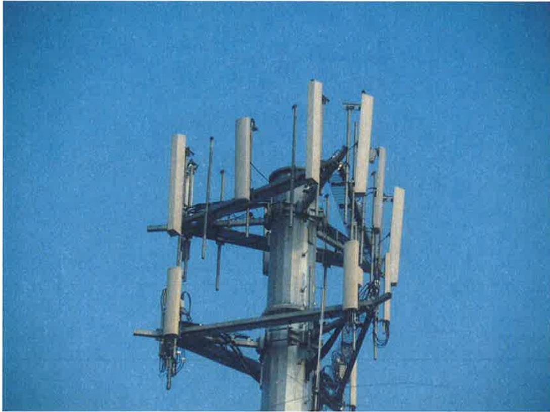
Photo 1: Photo illustrating the monopole with Appurtenances shown.
