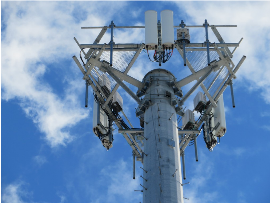
Photo 1: Photo illustrating the Monopole with Appurtenances shown.
