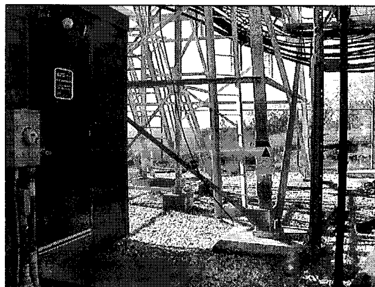
Nextel shelter (left); RF sign on tower leg
