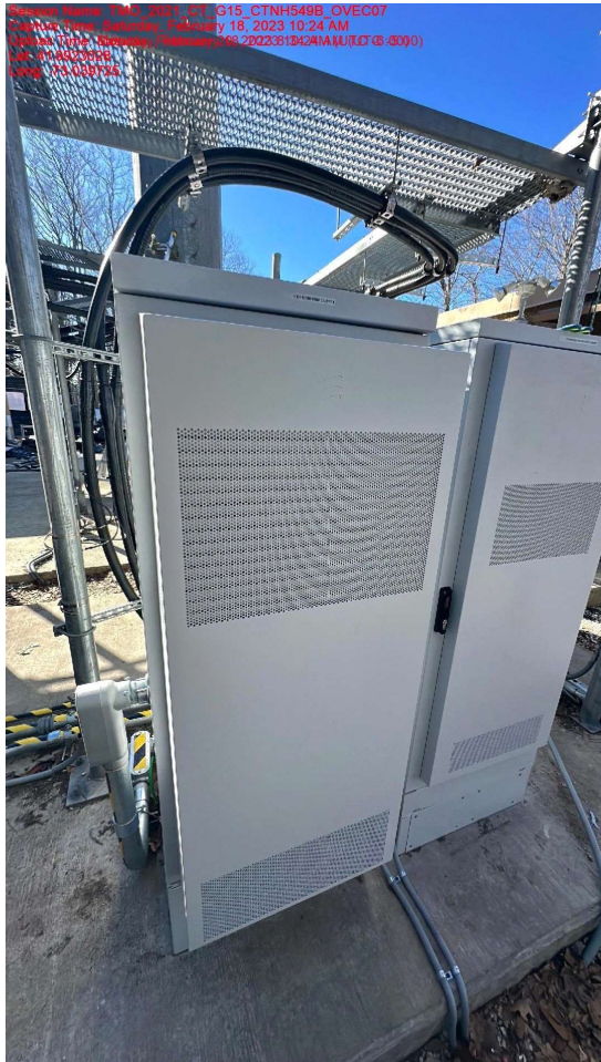
New Equipment Cabinet Mounted To Existing Concrete Pad
