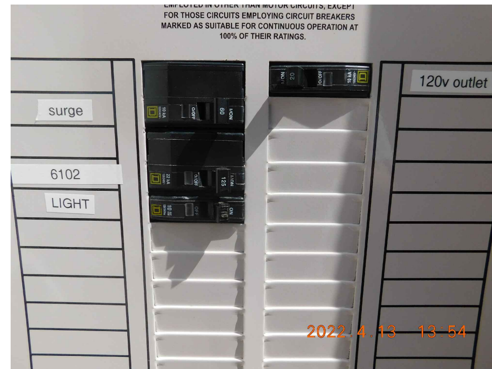
EXISTING POWER PANEL PHOTOS 1 SCALE: NOT TO SCALE E-1
