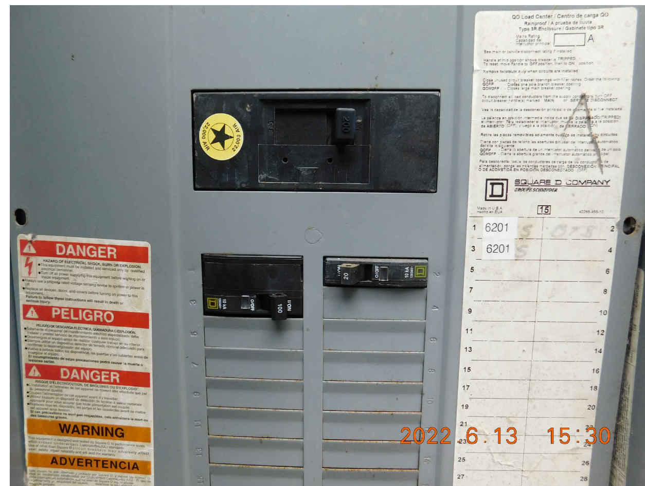
EXISTING POWER PANEL PHOTOS SCALE: NOT TO SCALE
