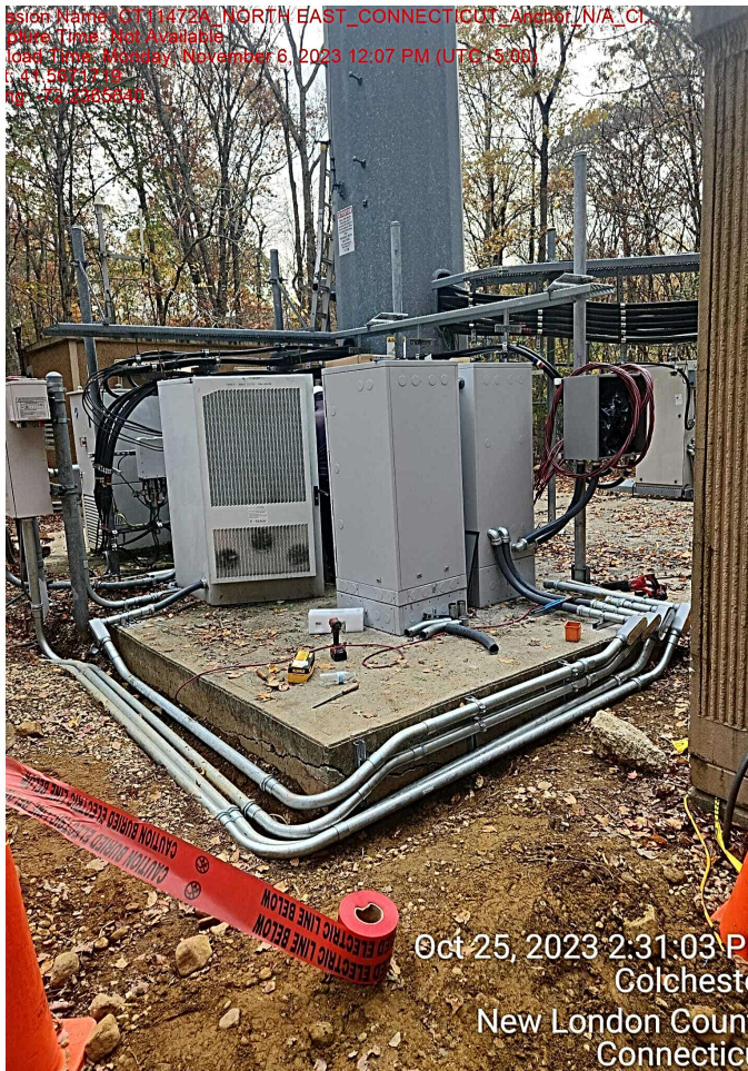
New cabinets installed on existing concrete pad
