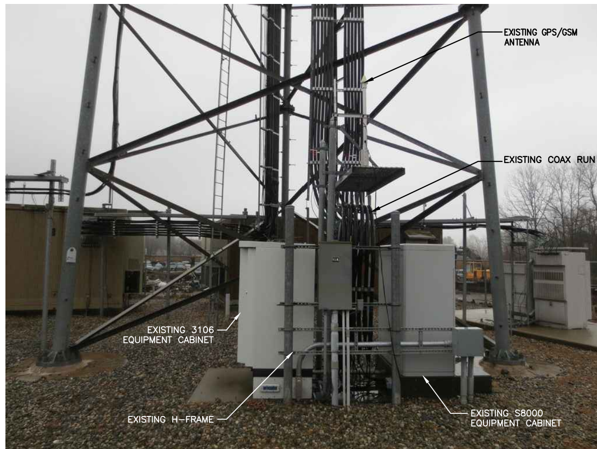
3 EXISTING EQUIPMENT PHOTO DETAIL
