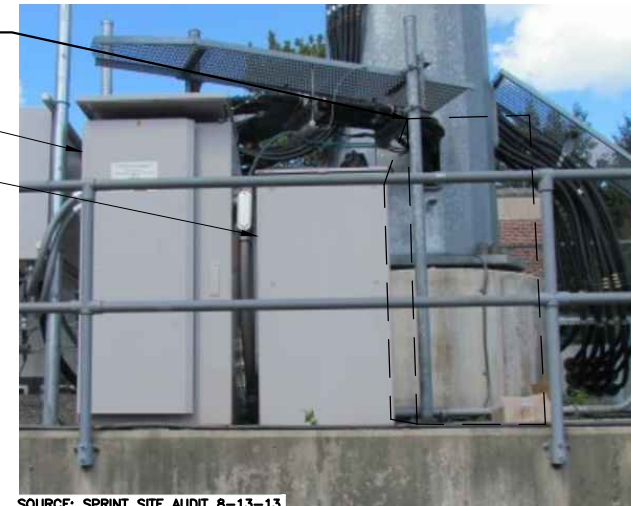
RAN EQUIPMENT PHOTO DETAIL SCALE: N.T.S.
