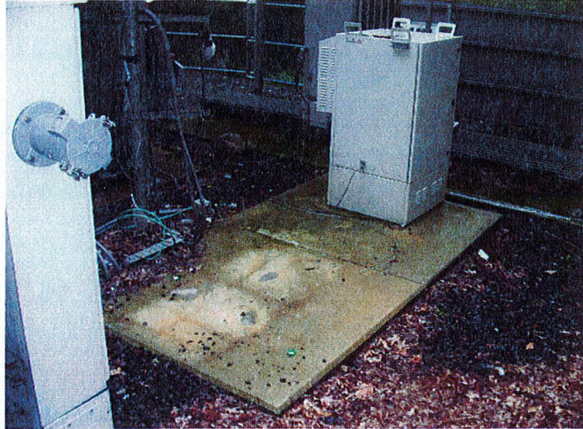
AT&T GROUND EQUIPMENT TO BE REMOVED
