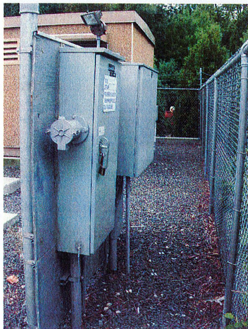
AT&T AC & TELEPHONE EQUIPMENT TO BE REMOVED
