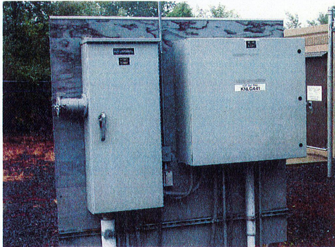
AT&T AC & TELEPHONE EQUIPMENT TO BE REMOVED
