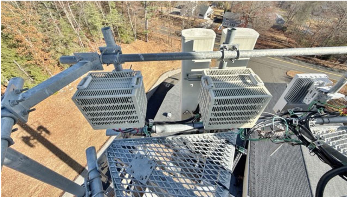
Fig. 1: Overall View of Antennas & Equipment (Alpha Sector)
