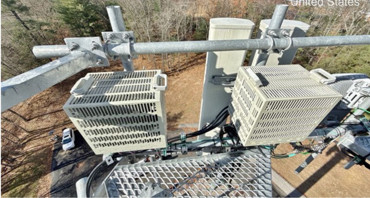
Fig. 3: Overall View of Antennas & Equipment (Gamma Sector)
