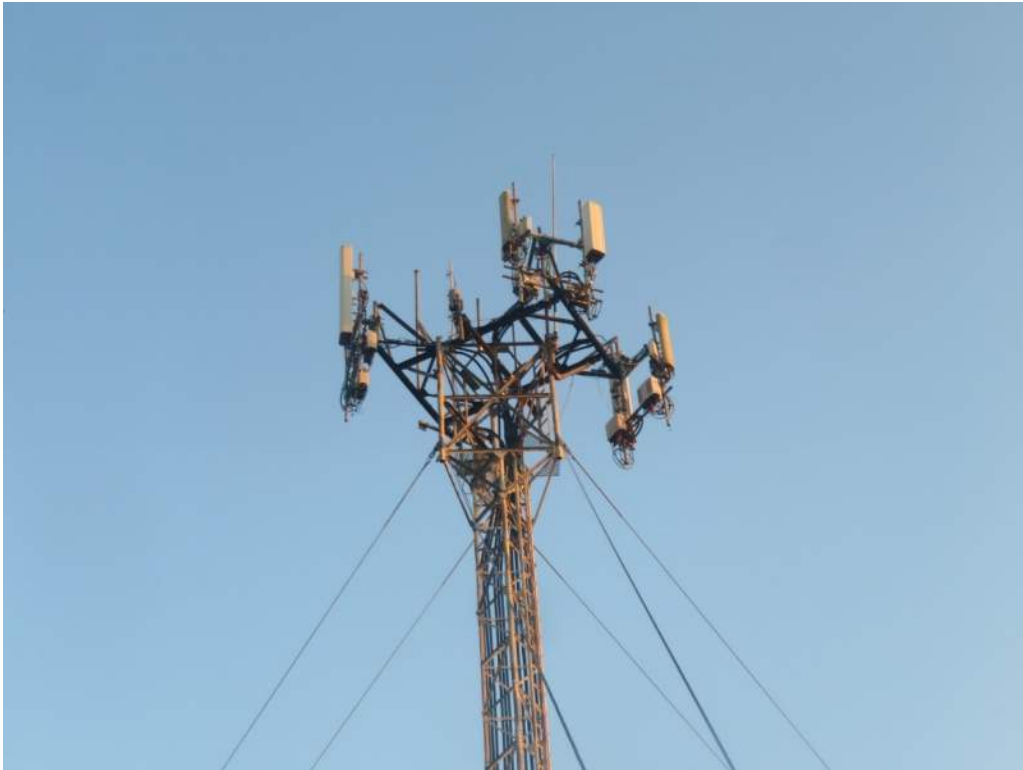
Photo 1: Photo illustrating the Tower with Appurtenances shown.
