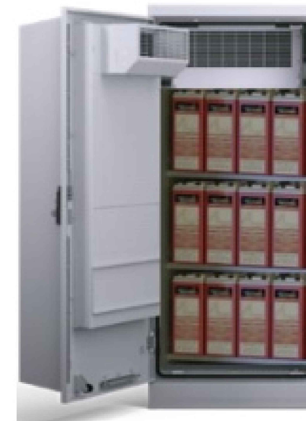
ERICSSON B160 EQUIPMENT CABINET
