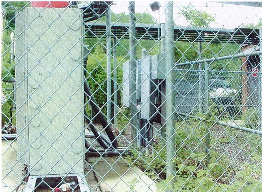
AT&T TELEPHONE & ELECTRICAL FIXTURES TO BE REMOVED (Shown located along fence on right)
