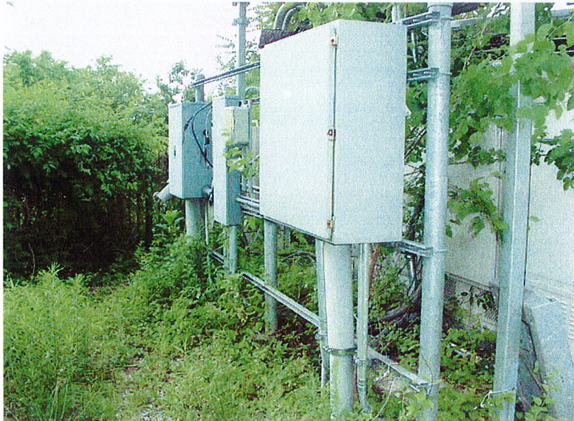
AT&T ELECTRICAL & TELEPHONE EQUIPMENT TO BE REMOVED
