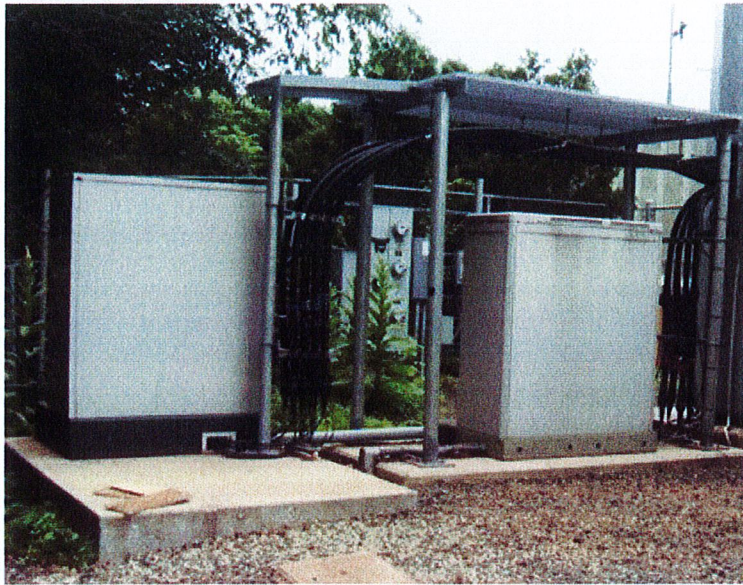
AT&T CABLE ENTRY TO SHELTER AND ASSOCIATED EQUIPMENT
