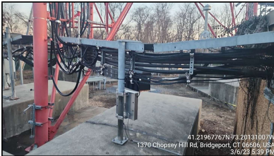
Figure 6: View of installed fiber and DC trunks in ice bridge
