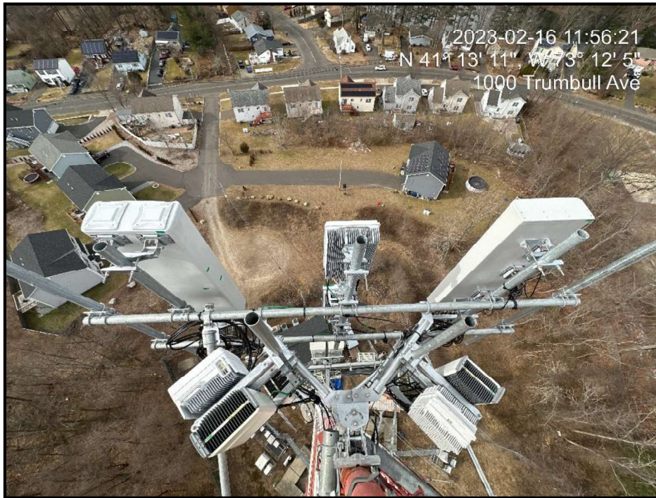
Figure 3: View of installed gamma sector antennas and RRUs on new sector frame
