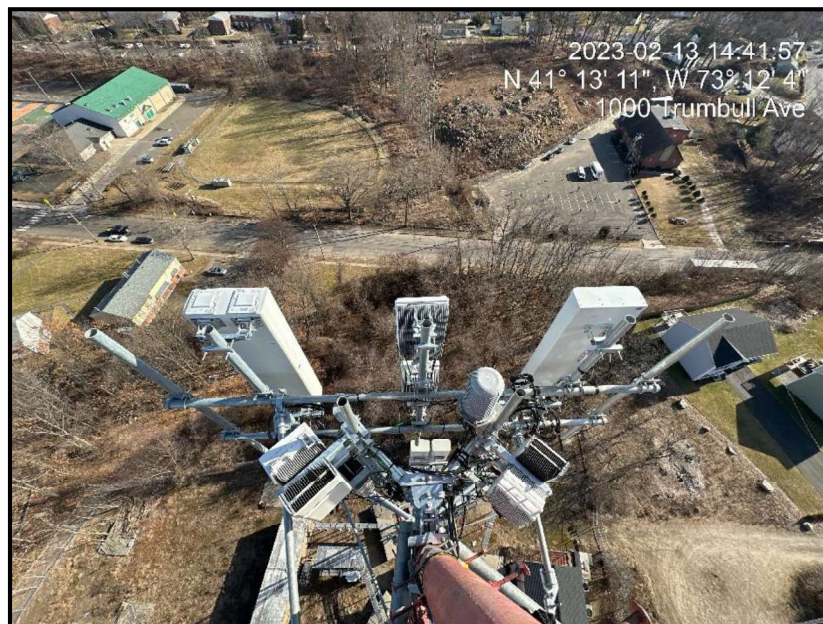
Figure 2: View of installed beta sector antennas and RRUs on new sector frame
