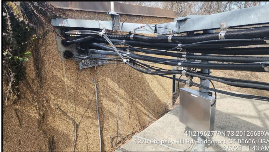
Figure 5: View of installed fiber and DC trunks in entry port
