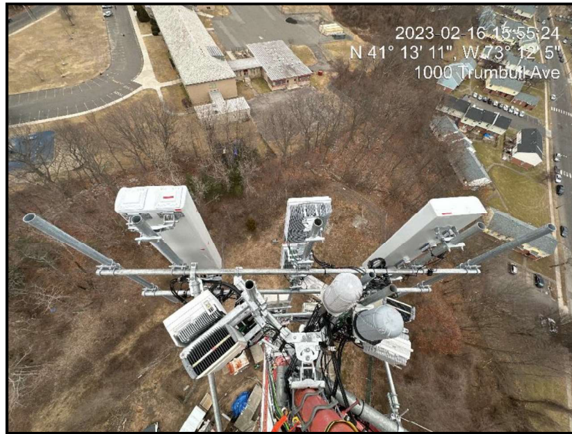
Figure 1: View of installed alpha sector antennas and RRUs on new sector frame
