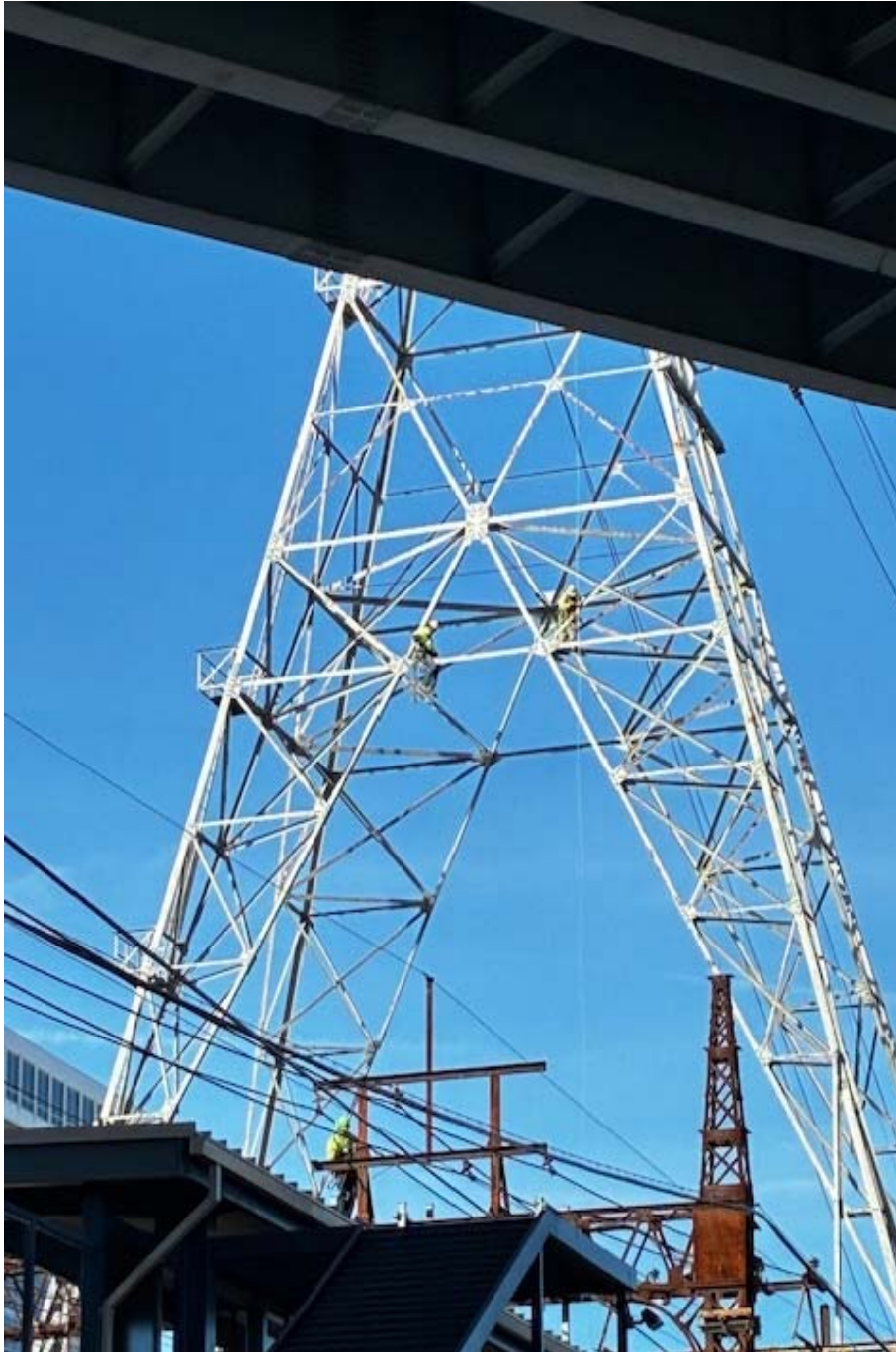
Picture 6 – UI crew using pulley system to lower the static wire from Structure 776
