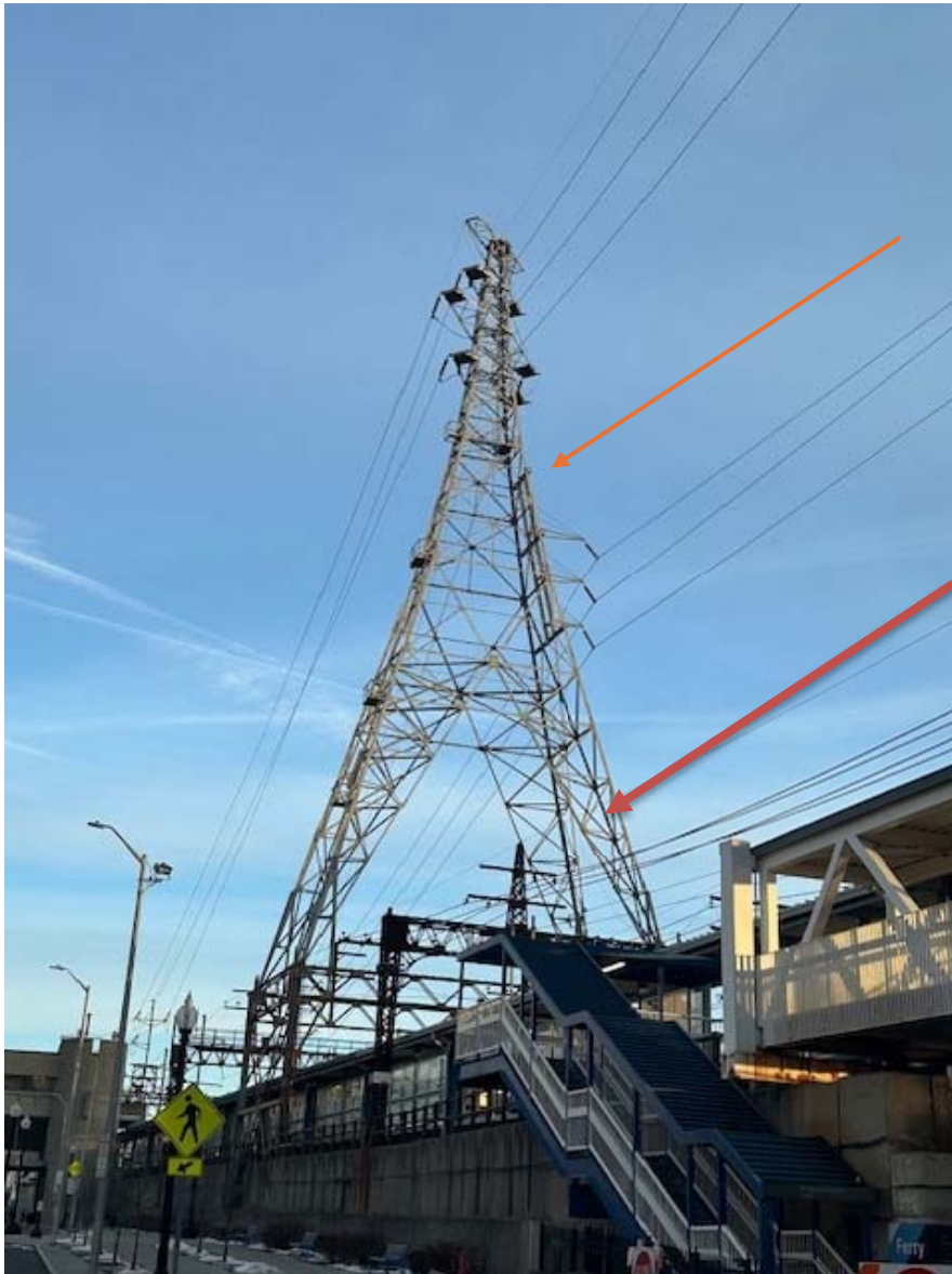
Picture 3 - Static hanging from atop Structure 776 onto and across MNR facilities and public areas
