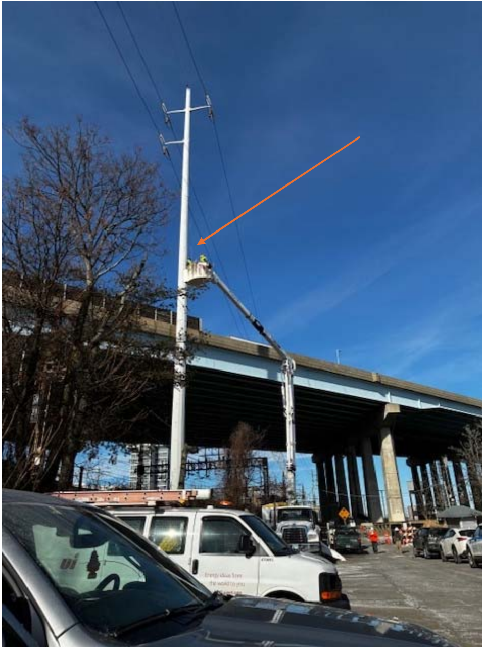
Picture 4 – UI crew affixing broken static to Structure P775B
