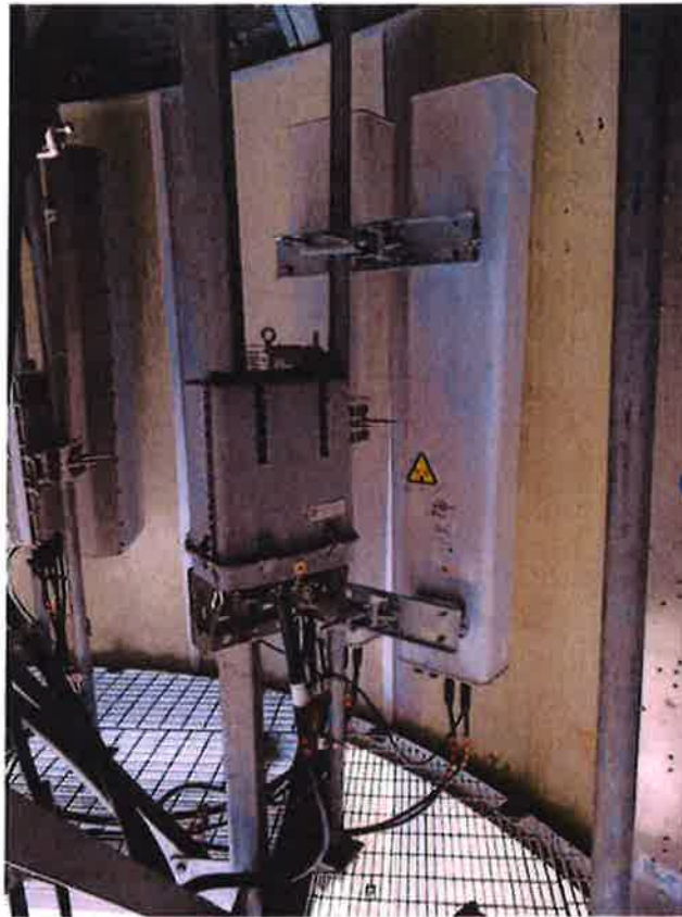
Photo 1: Sample photo illustrating existing antennas.
