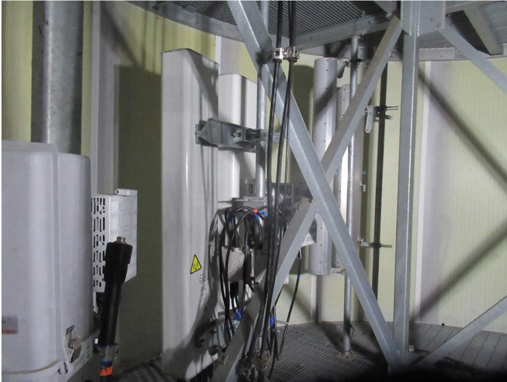
Photo 1: Sample photo illustrating existing antennas.
