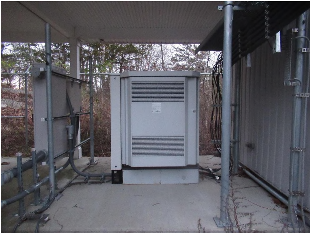
Photo 2: Sample photo illustrating existing equipment located under canopy.
