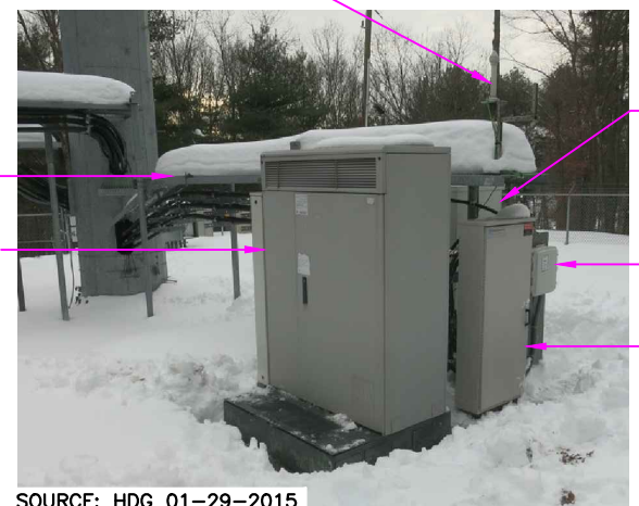
EQUIPMENT PHOTO DETAIL (3/A-1) SCALE: N.T.S.
