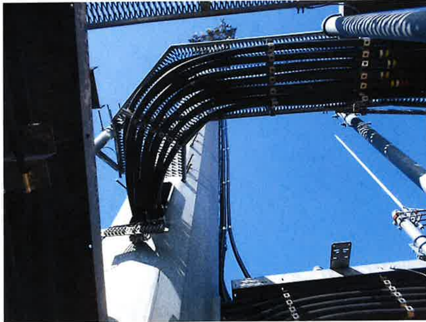
Photo of existing feed lines and ground bars at tower.
