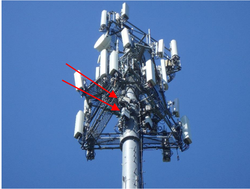
Figure #3 – View of installed Beta sector AT&T RRUS (typical).
