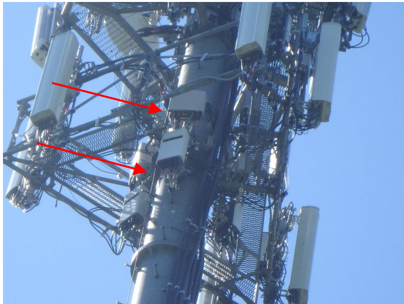
Figure #4 – View of installed Gamma sector AT&T RRUS (typical).
