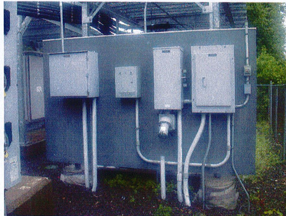
AT&T AC & TELEPHONE EQUIPMENT TO BE REMOVED
