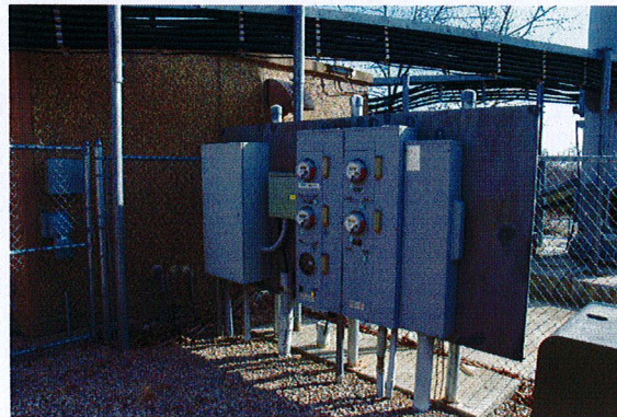
FORMER AT&T AC & TELEPHONE EQUIPMENT AREA
