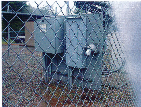
AT&T AC & TELEPHONE EQUIPMENT TO BE REMOVED
