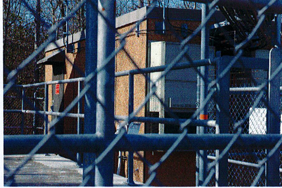
FORMER AT&T SPACE CLEARED OF EQUIPMENT
