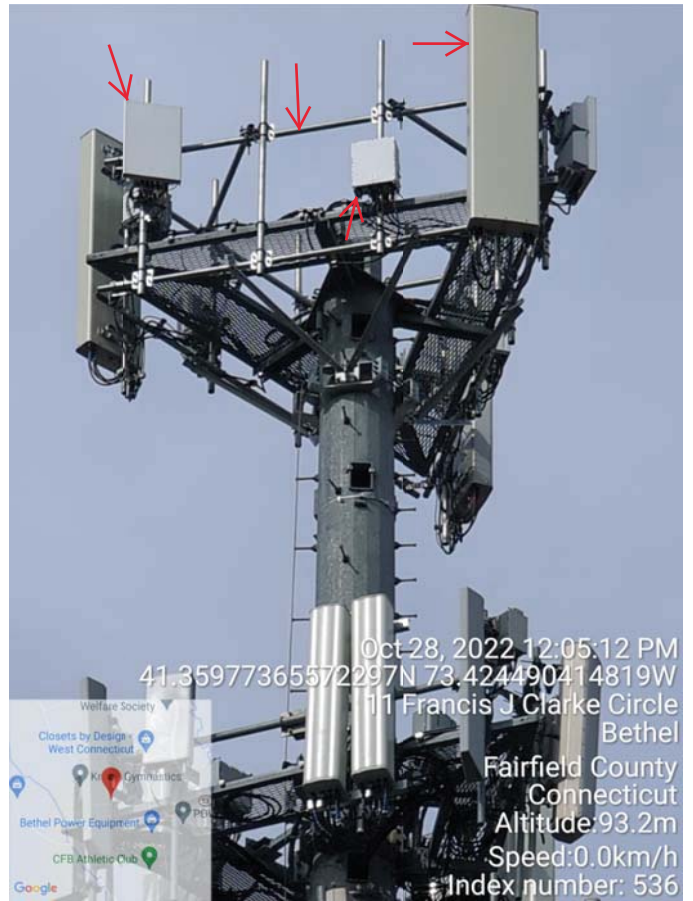
Alpha Sector: (2) New Antennas & (2) New RRH Mounted To Existing Platform with New Handrail Kit On Existing Monopole
