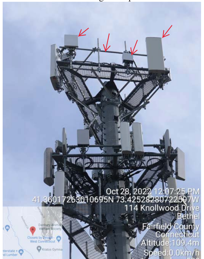
Gamma Sector: (2) New Antennas & (2) New RRH Mounted To Existing Platform with New Handrail Kit On Existing Monopole
