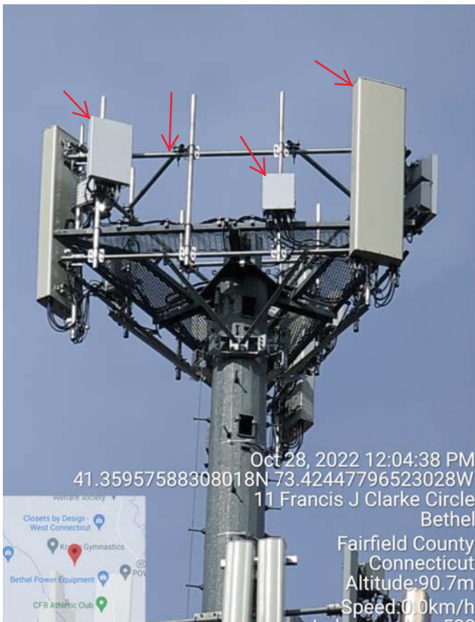
Beta Sector: (2) New Antennas & (2) New RRH Mounted To Existing Platform with New Handrail Kit On Existing Monopole
