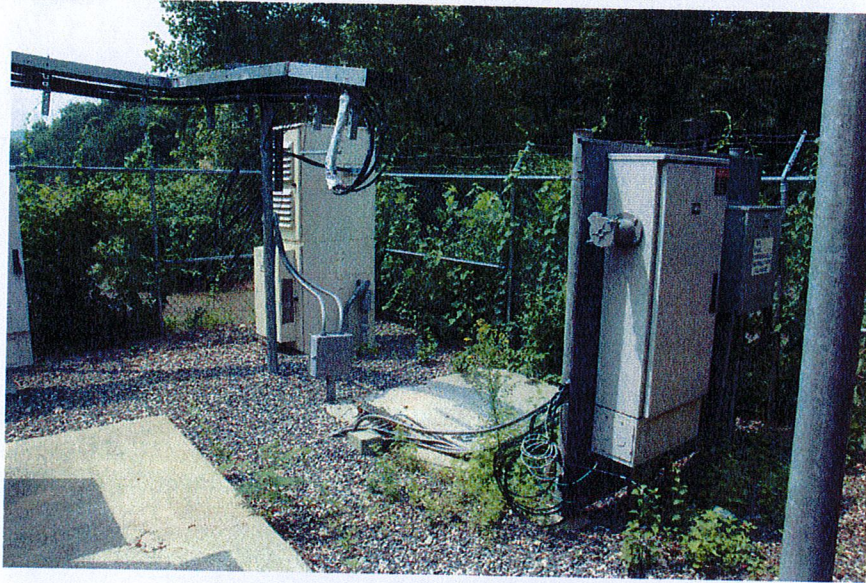
AT&T BASE STATION AND ASSOCIATED EQUIPMENT
