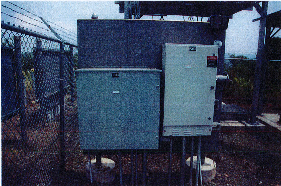
AT&T ELECTRICAL AND TELEPHONE EQUIPMENT
