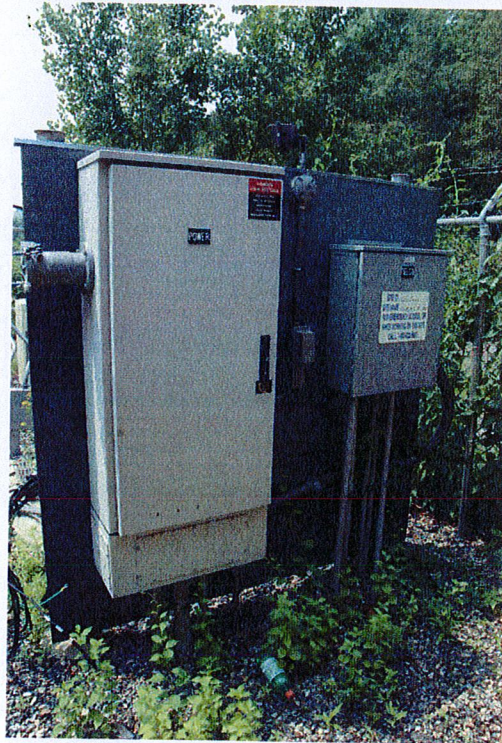
AT&T ELECTRICAL AND TELEPHONE EQUIPMENT
