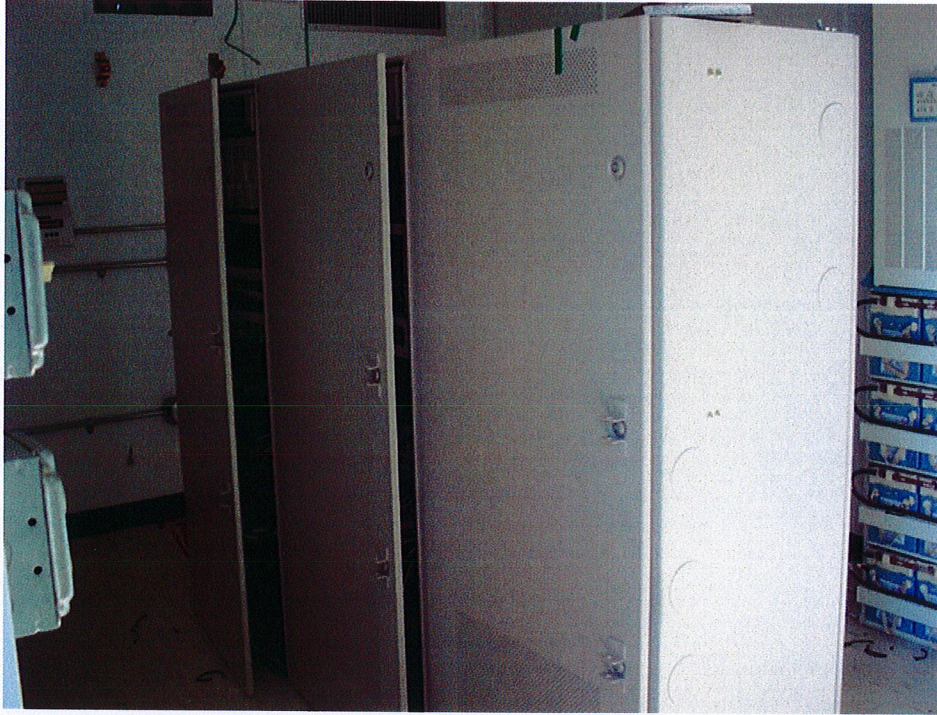
AT&T Ground equipment before removal
