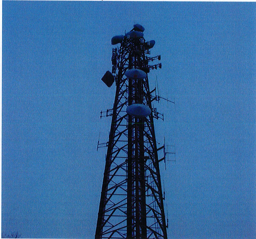
AT&T Array to be removed (2 nd from bottom)
