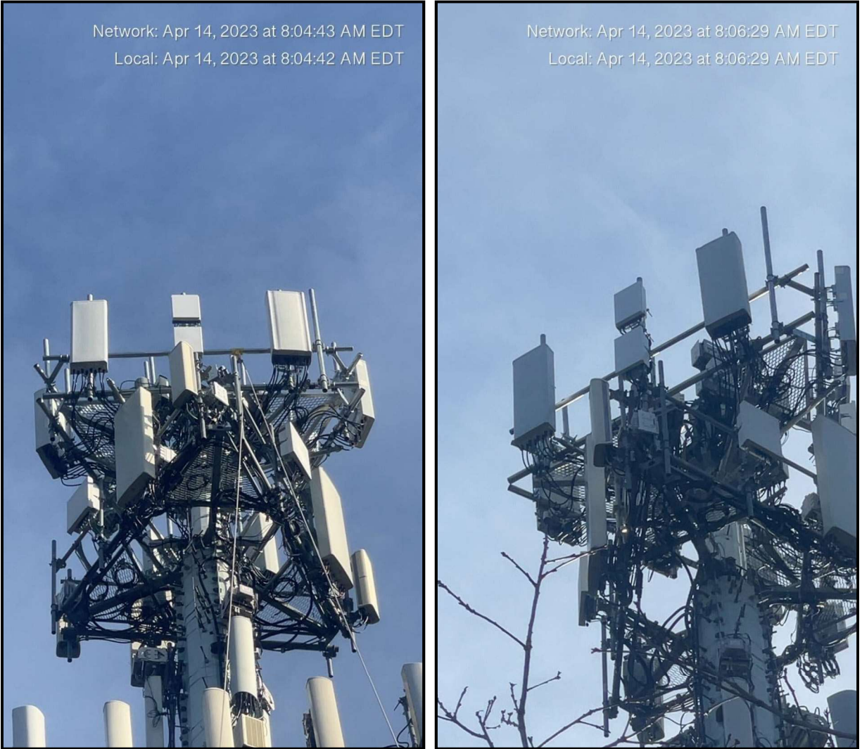
Figure 3: Overview of installed equipment on tower
