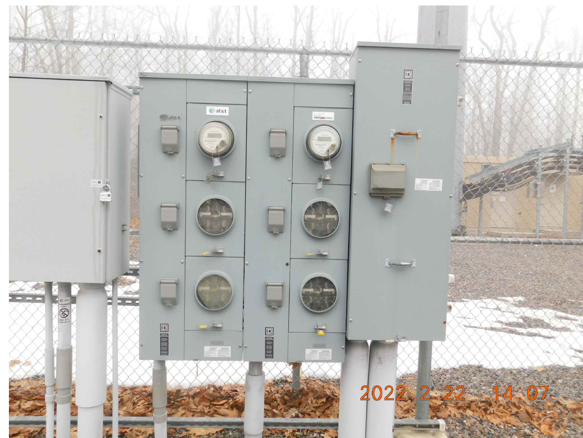
EXISTING METER BANK PHOTO 6 E-1 SCALE: NOT TO SCALE
