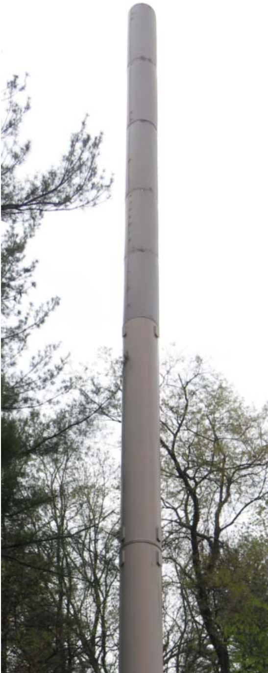
Exhibit A: Existing T-Mobile Mount (Behind Shroud) Photo Date 05/03/2019
