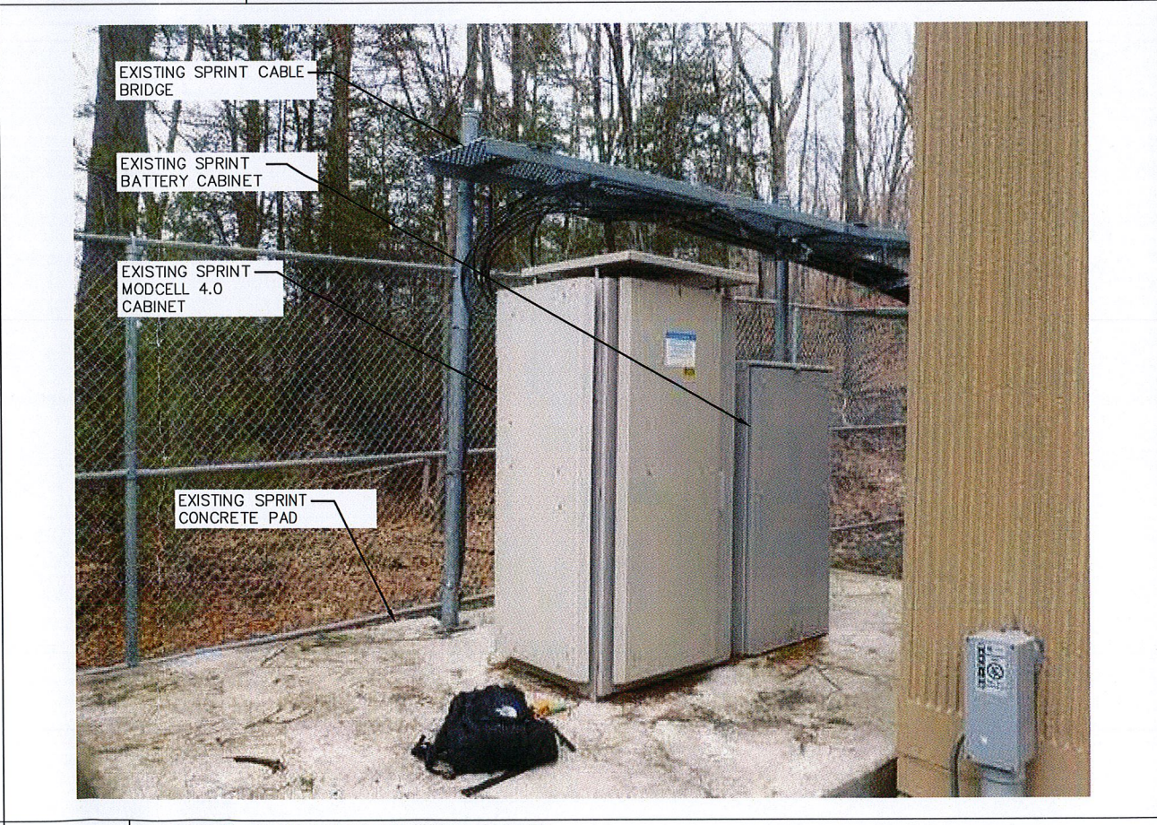
4 EXISTING EQUIPMENT PHOTO DETAIL SCALE: NTS
