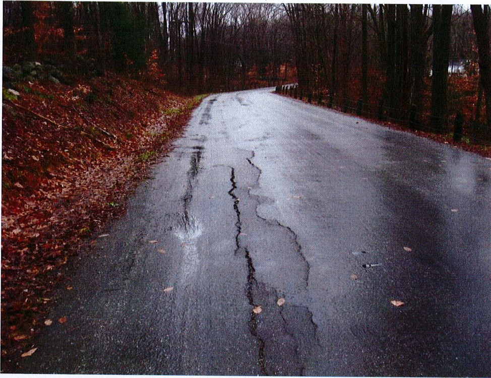
Flagg Hill Road – Longitudinal Cracking
