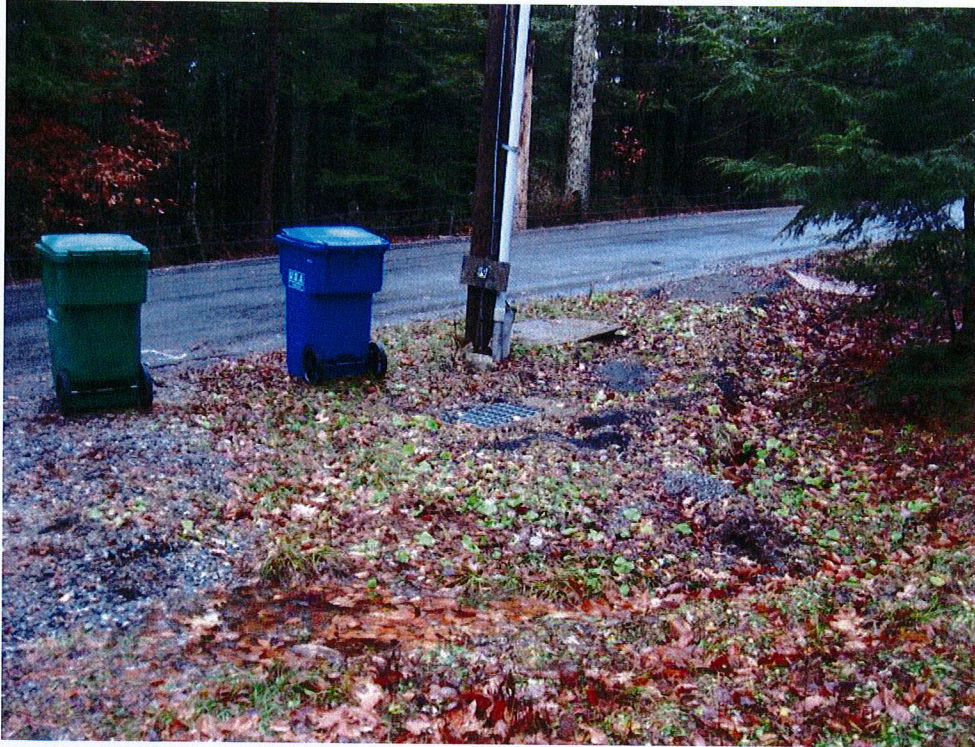
Gravel Driveway on Flagg Hill Road – Erosion due to poor drainage
