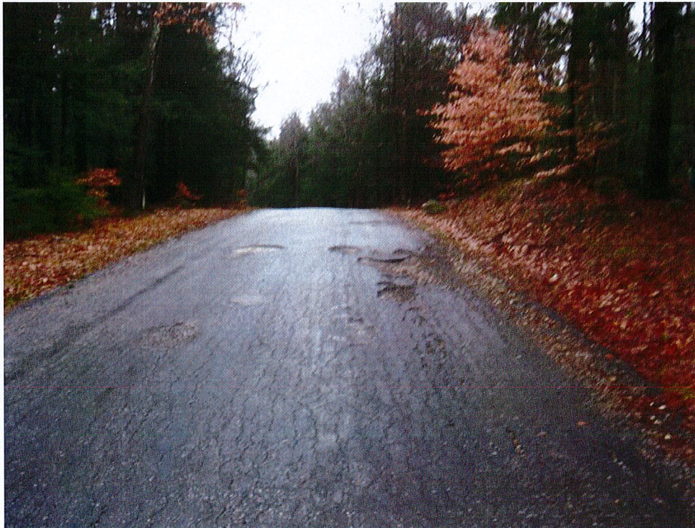
Rock Hall Road – Potholes and Pavement Cracking
