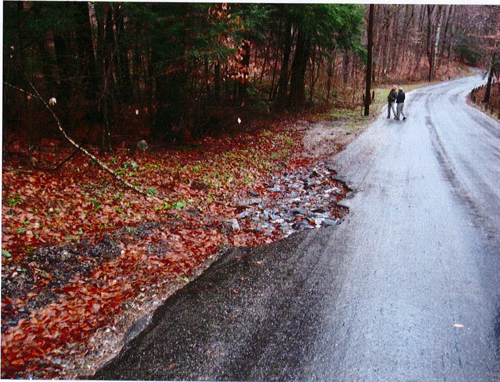
Flagg Hill Road – Area of Pavement Failure
