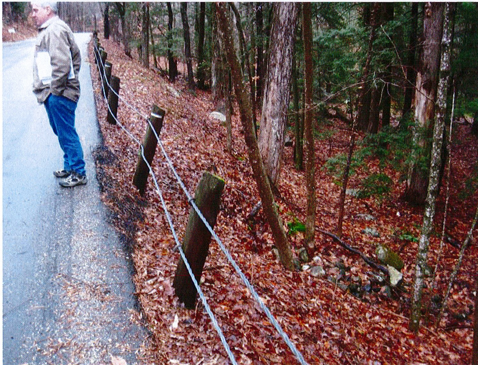
Flagg Hill Road – East Side, sheet flow and steep fill slope
