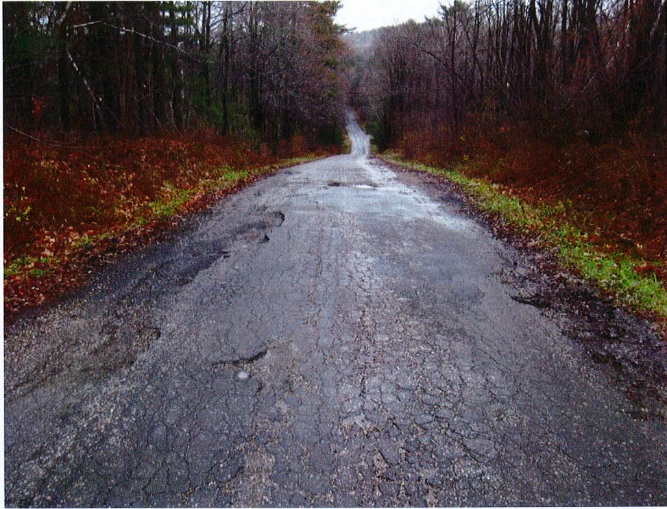
Rock Hall Road – Potholes, Pavement Failure Area, Pavement Cracking
