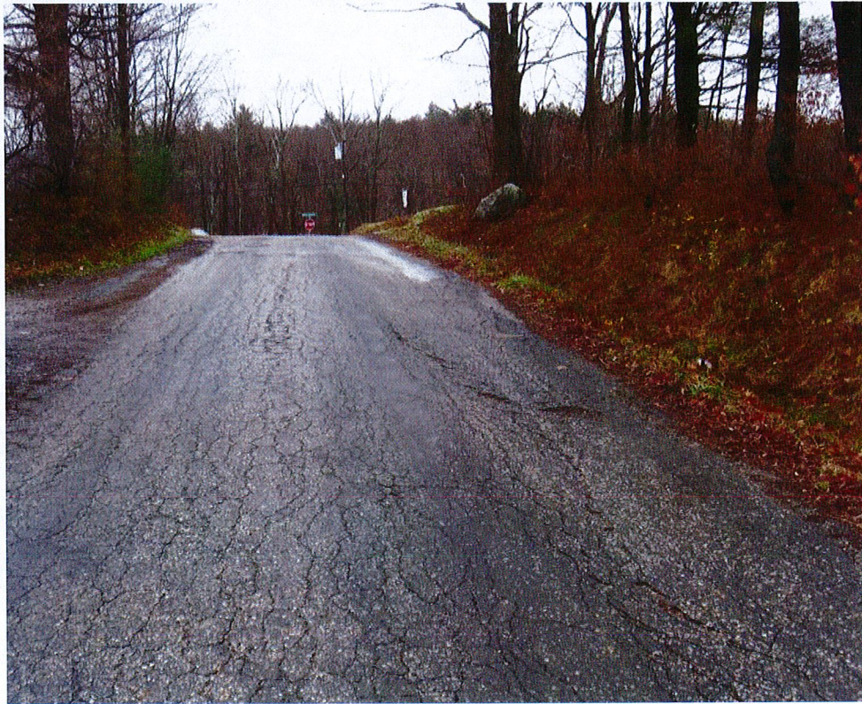
Rock Hall Road – Alligator Cracking, Rutting on Roadway Edge
