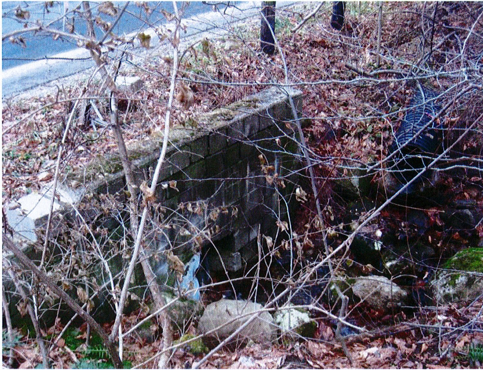
Flagg Hill Road – CMU Headwall and culvert with contributing pipe, West Side
