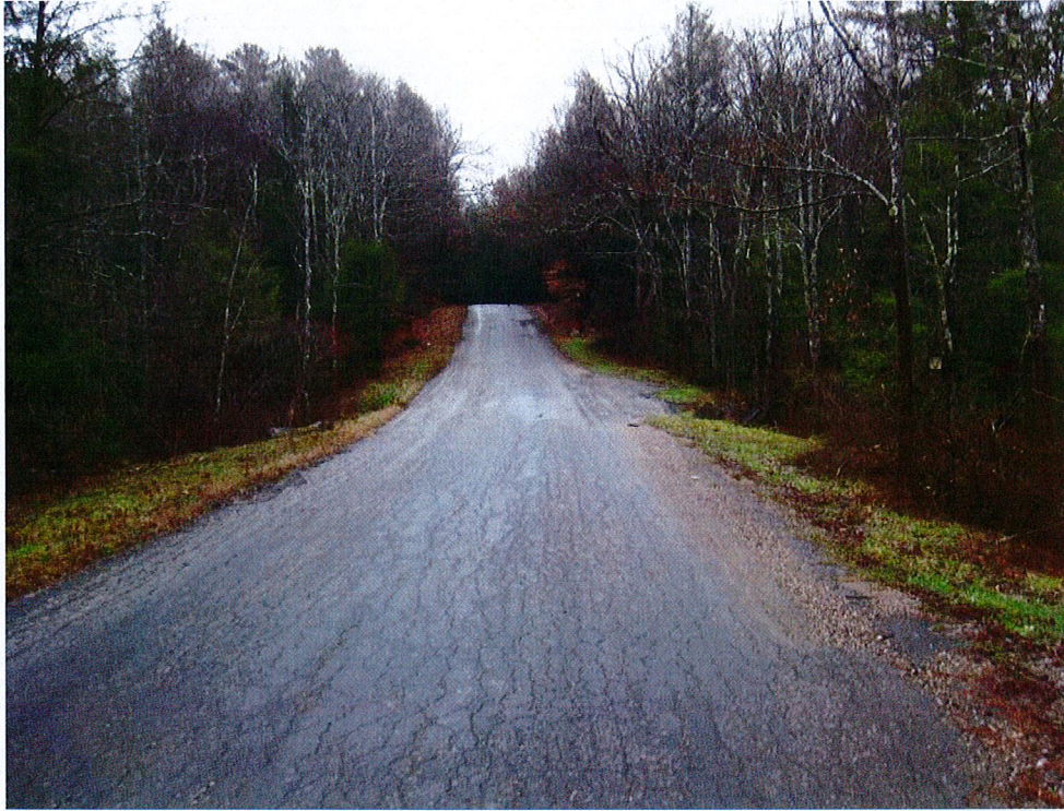
Rock Hall Road – Alligator Cracking
