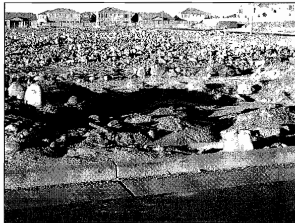
Blobs of concrete washout material next to a washout pit. Most likely a result of washing out pump trucks.
