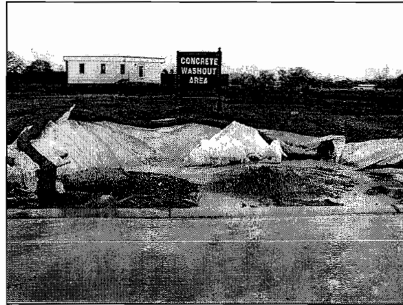
An inadequately maintained and constructed concrete washout pit. Hazardous wash water is allowed to overflow the curb and eventually discharge into the storm drain.
