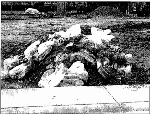
A pile of plastic washout bags on a jobsite. Each bag was broke, which allowed caustic washwater to escape
