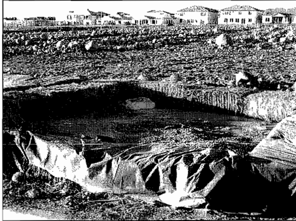
A washout pit that does not comply with local BMP's as the plastic is torn and not covering the hay bales to prevent leakage.
