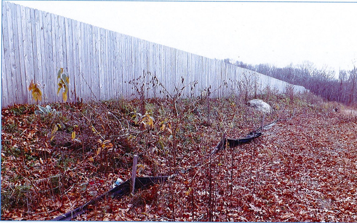
Southwest section of project site. Nonfunctional silt fencing. Landscaping specified in this area.
