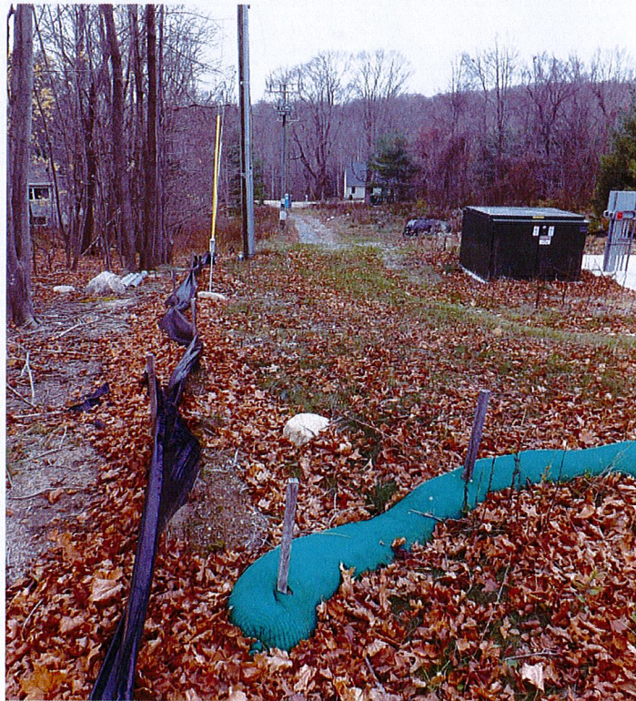
Silt fence, silt socks and discarded PVC pipe along electrical connection corridor.
