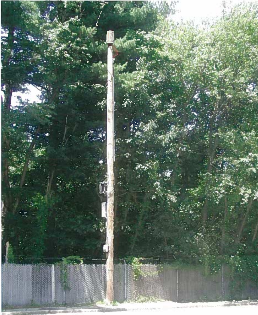
Figure 20 - DAS Node in Brookline, Massachusetts
