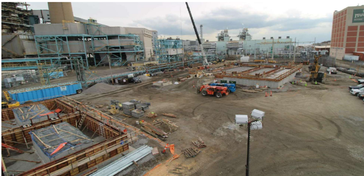
Photo 1: Broadview of project site with TXF and GIS foundation walls being installed.
