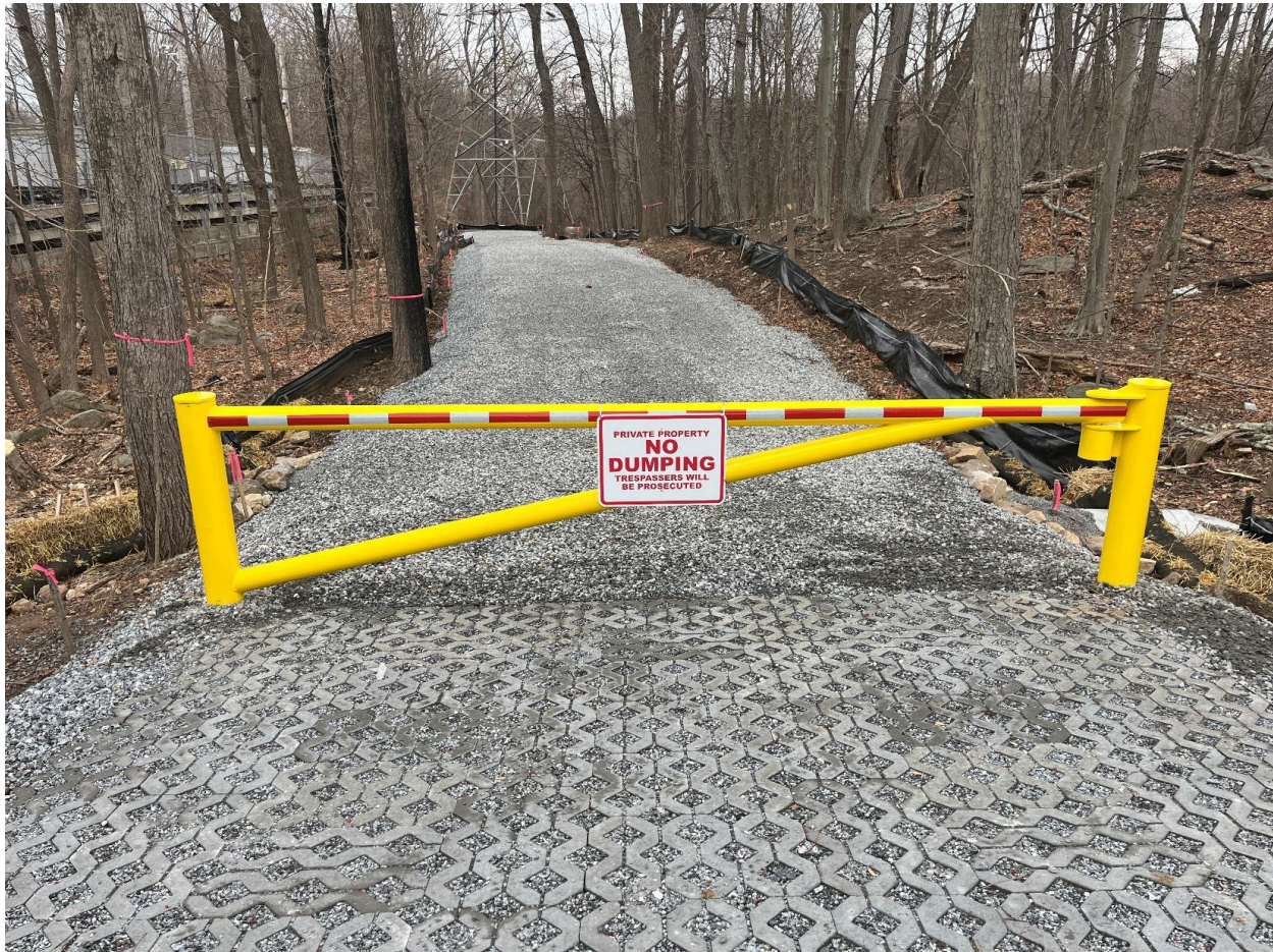
Photo 1: View of the newly installed access gate at the southwestern access road.
