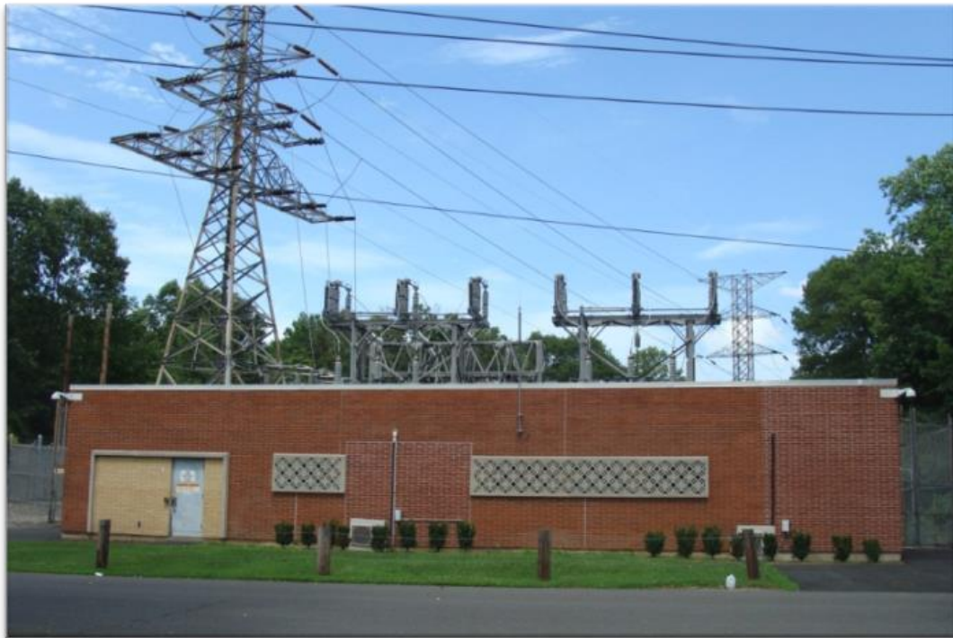
Figure 1-3: Street-Level View of Existing Old Town Substation (Looking East from Kaechele Place)
