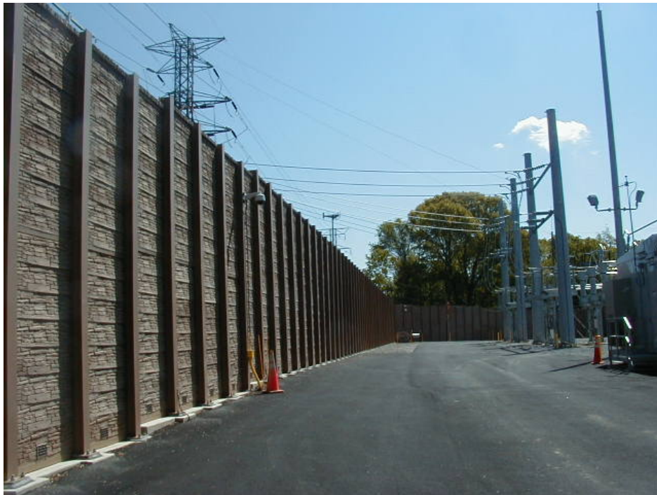
Figure A-4. Interior view of Trumbull substation north wall facing tap structures.
