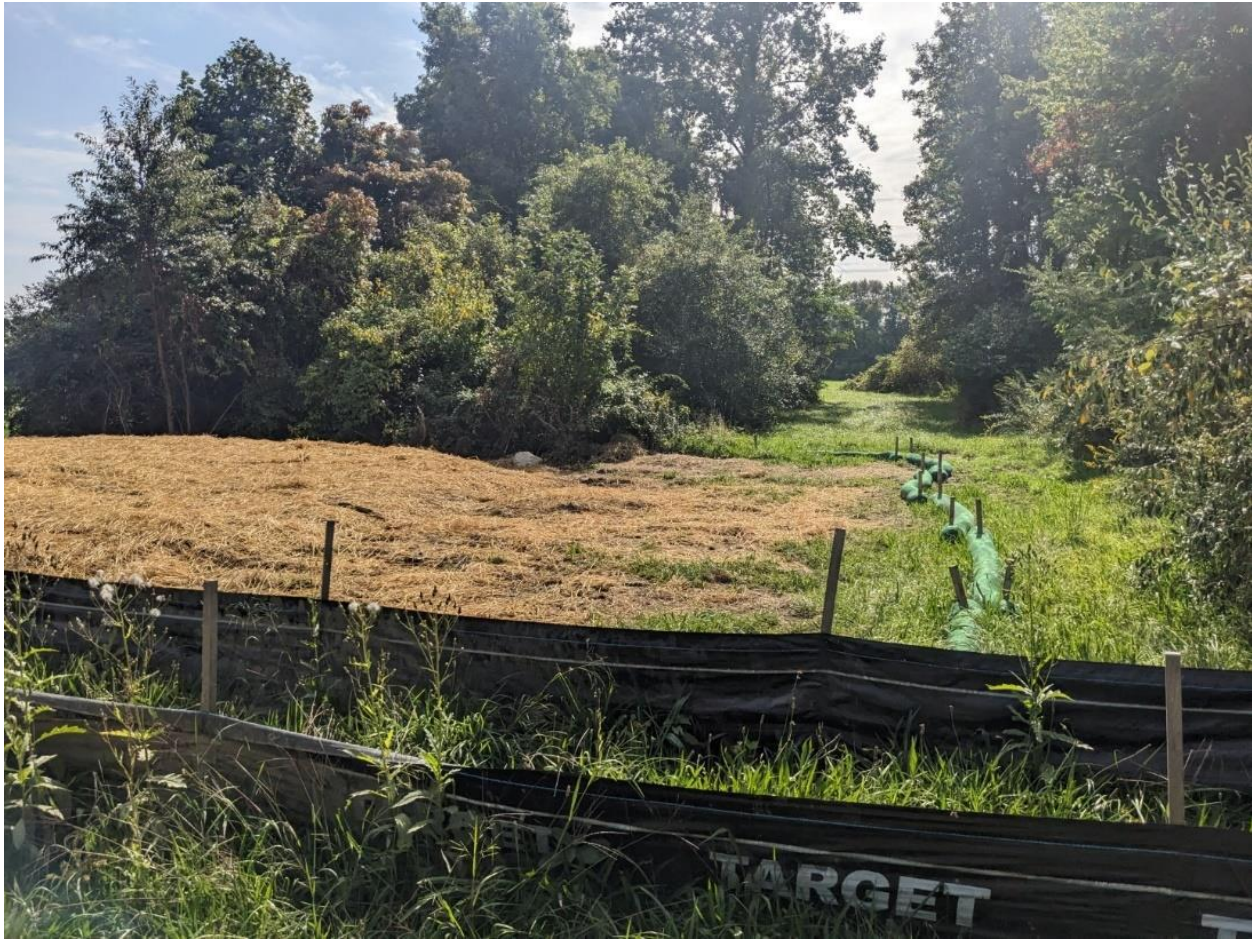
Photo 2: Material spread between STR 351 and STR 352, and stabilized with seed and straw.
