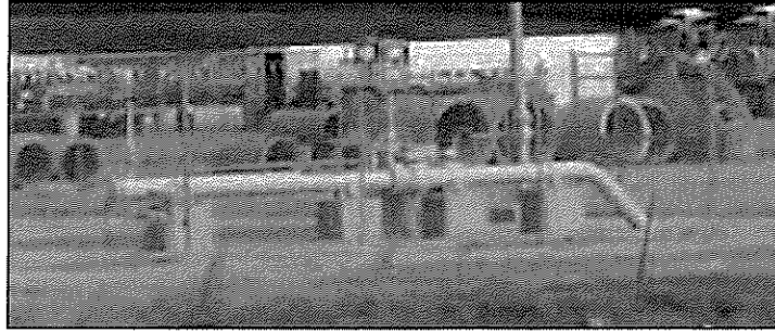
Figure 2-4 Gas Yard Pigging Station Receiver/Launcher
