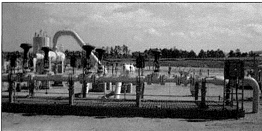
Figure 2-5 Typical Gas Yard Pressure Regulators
